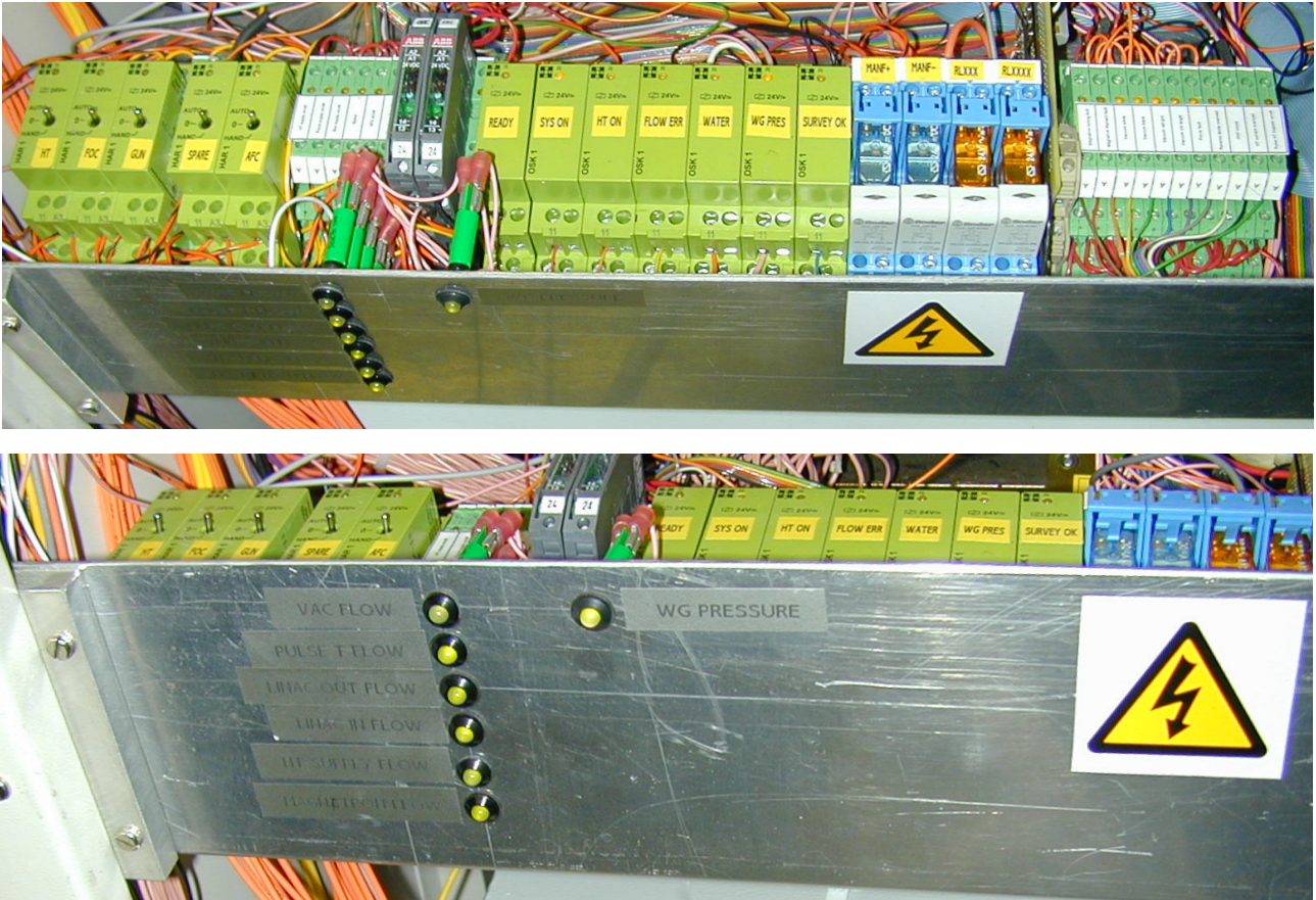
Figure 5: Practical arrangement of opto-isolators and relays on DIN rail; Flow and waveguide pressure switches can be seen in the lower image.
